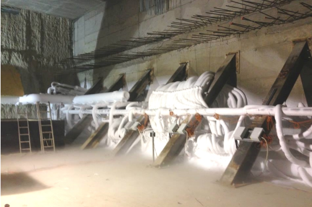
Liquid nitrogen installations - West Shaft
